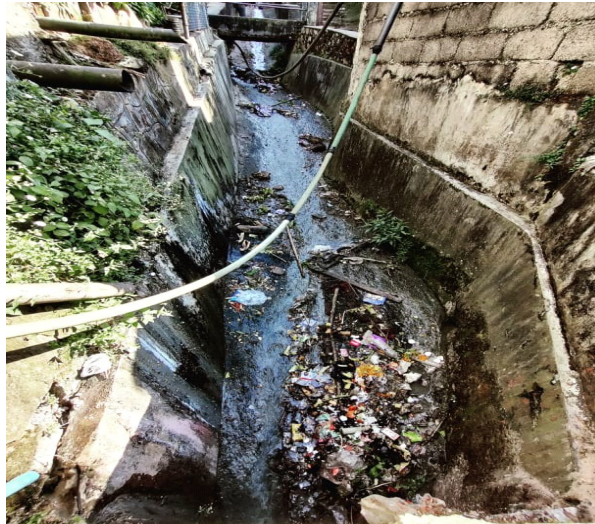
Plate 3: Illegal Dumping of solid Waste in drains flowing to Umshyrpi River.
